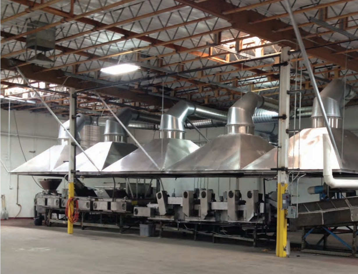
Five custom collection hoods built over the processing line to capture odor and smoke are ducted to the Smog-Hog unit outside.
